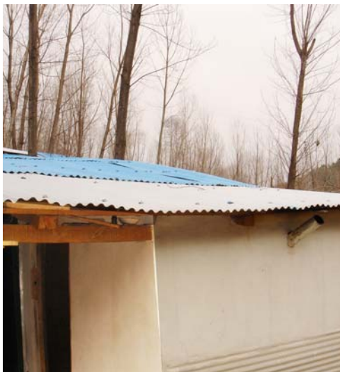
A view of completed kitchen at one of shelter at Village Bermong
